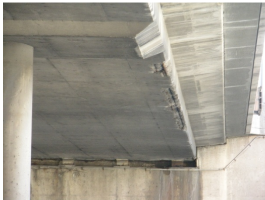
Spalls along West Face
