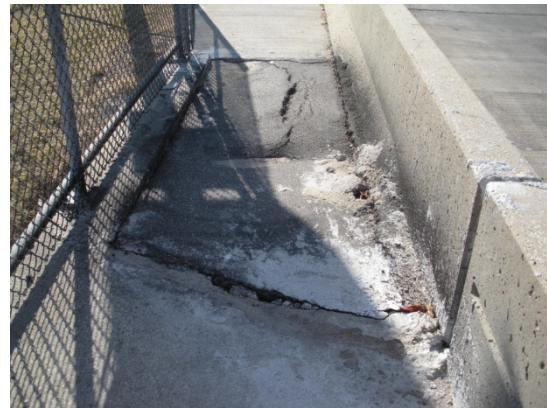
Settlement of Sidewalks at Approach Slab
