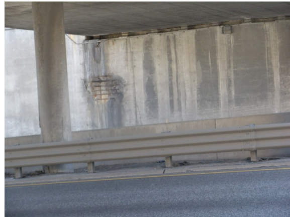
Large Spall in South Abutment
